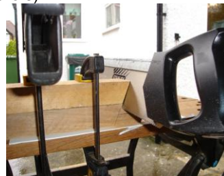
Picture 3 - The 2nd cut. Note the use of clamps to hold the two legs in position. Hold the side of the saw blade against the 70° angled edge of the top leg while cutting.
